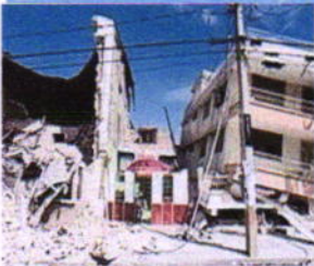
(Building crashed in Port-au-Prince)
